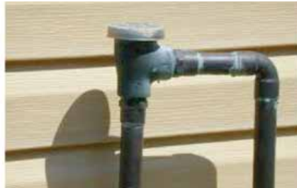
Atmospheric-type Vacuum Breaker
